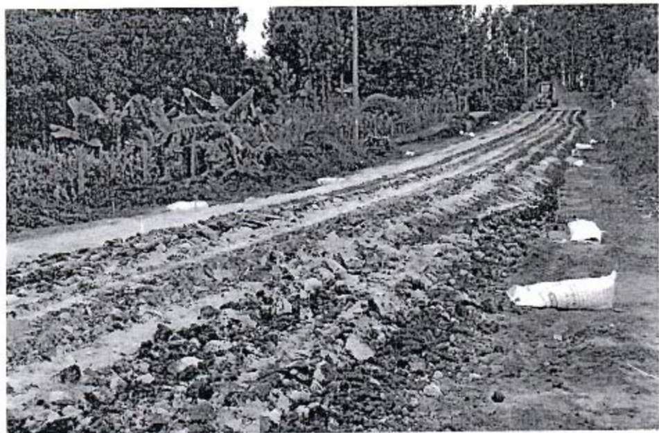
Photo 5: A section of the road being worked on by the contractor. Special Vardener is used to help in compacting the 11th bats.
