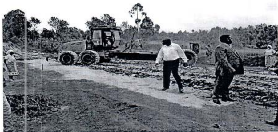
Photo 4: The Chairman and Vice Chair to the committee inspect a section where the process of soil stabilization was being undertaken.
