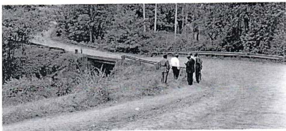
Photo 6: Ndanda bridge- it's a narrow and has very sharp bends on both sides.
